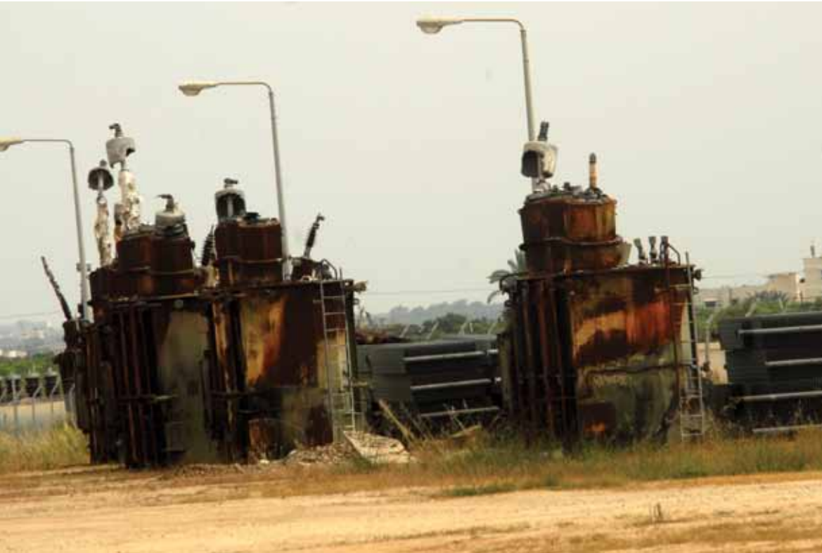
The Gaza power plant was damaged after being bombarded by Israeli forces. (2009)
